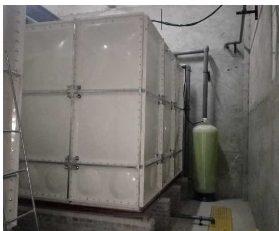
活性炭吸附罐
